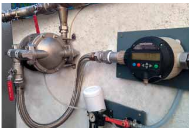
FMC 100 in combination with air-operated diaphragm pump for manual use.
