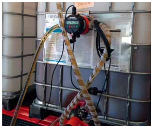
Semi-automatic filling with FMC 100 and switching amplifier FSV 100 from IBC.
